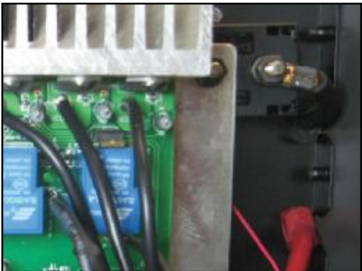
Circuit Breaker is fastened to the aluminum plate of the SCR board assembly.
